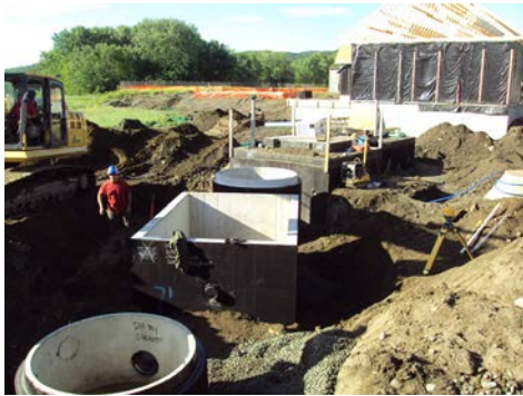
Installation of innovative septage receiving station
