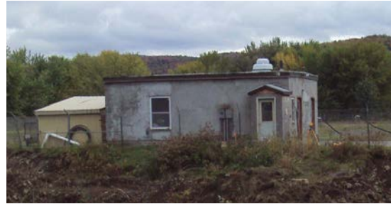
The existing control building was not in compliance with current safety regulations
