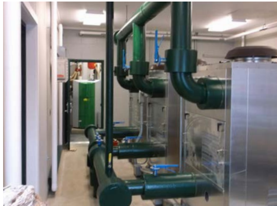
Enclosed VFD driven aeration blowers and insulated air piping for aerating of lagoons
