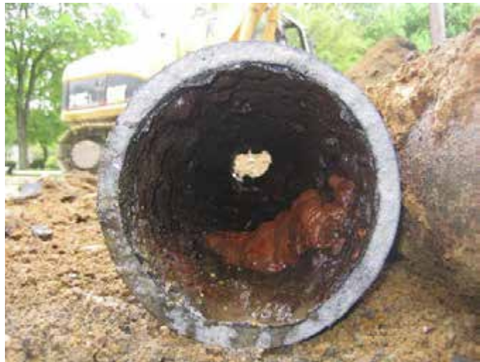
Tuberculation of water main
